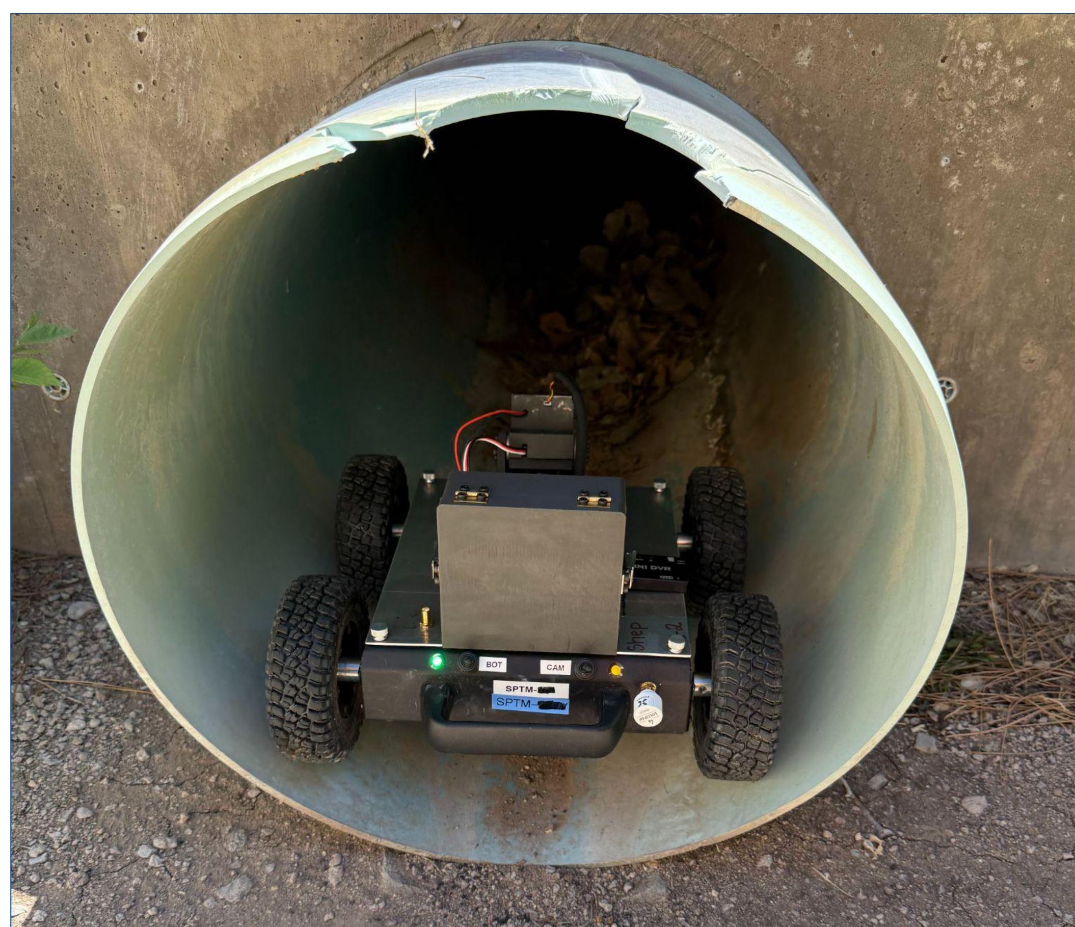
Figure 2. An image of the internal inspection system at the outlet of an 24" diameter HDPE culvert.
