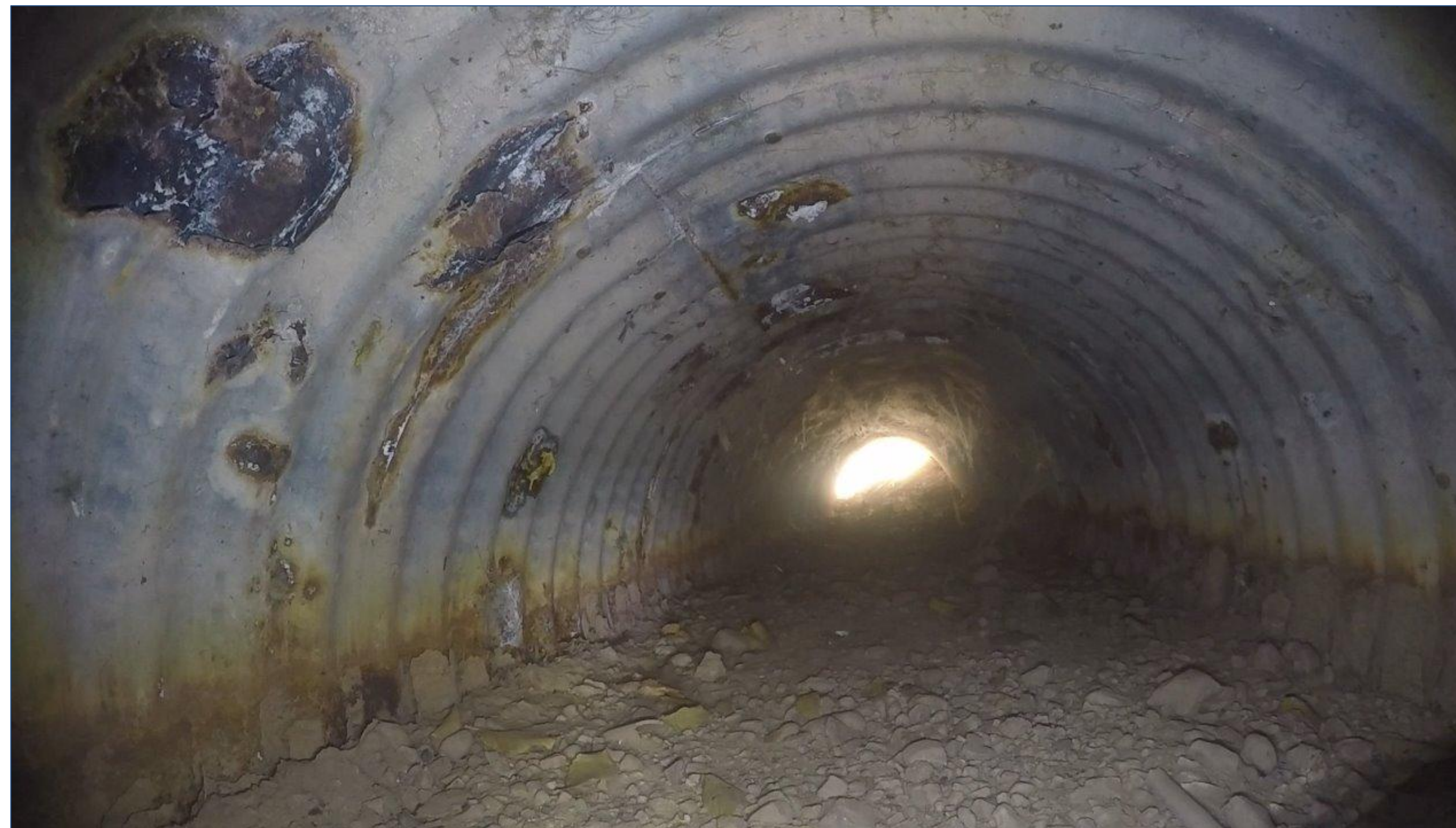
Figure 1. An internal view of an NM-based corrugated steel culvert with a moderate amount of silting and corrosion. Image was obtained via the inspection system.
